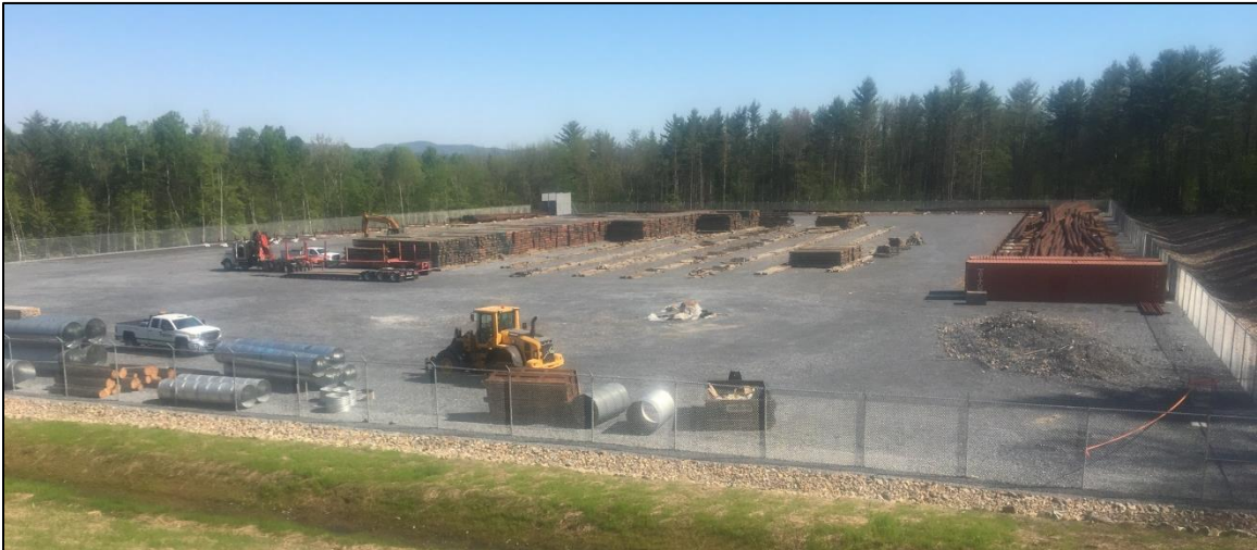
Photo 1: View of the recently constructed storage yard, looking north. The proposed building is to be located in the southeast corner of the yard.
